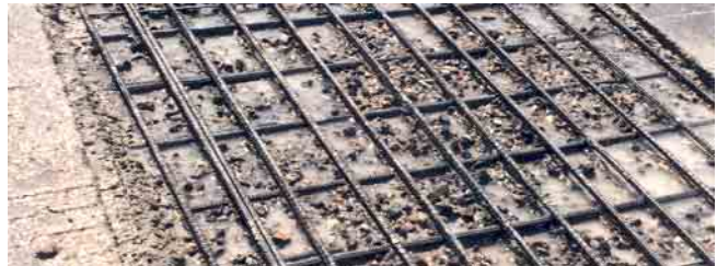
Hydrodemolition leaves rebar free of damage and clean for ideal new overlay bonding.
