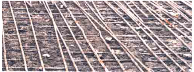
Damaged rebar grid on bridge deck after concrete removal with jackhammers.
