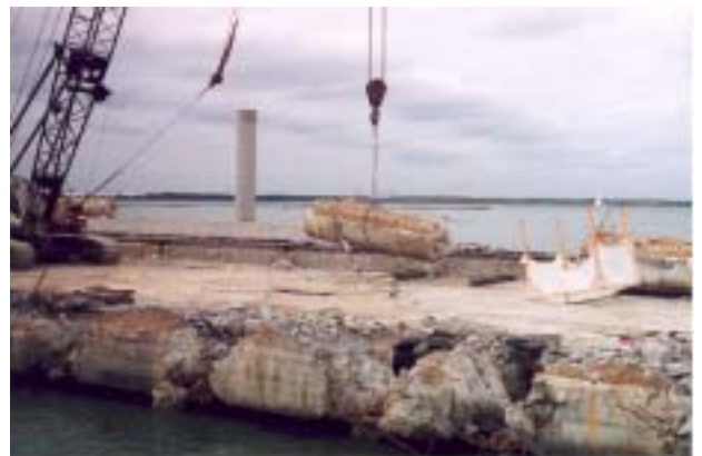
Once the concrete and steel was removed the beams were lifted away with a crane.
