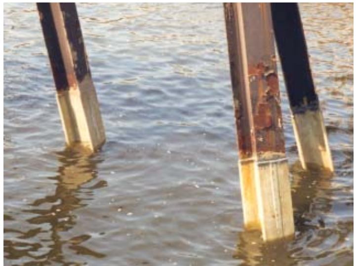
The fiberglass cladding is installed over the prepared surface and extends the life of the steel pilings.
