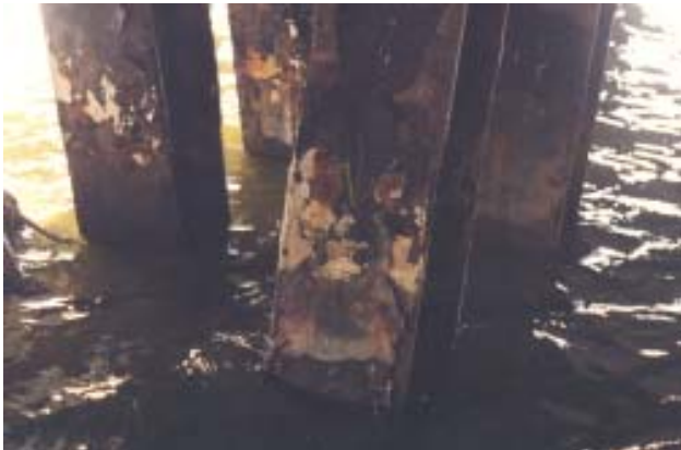
View of the steel pilings prior to application of the high-pressure water.
