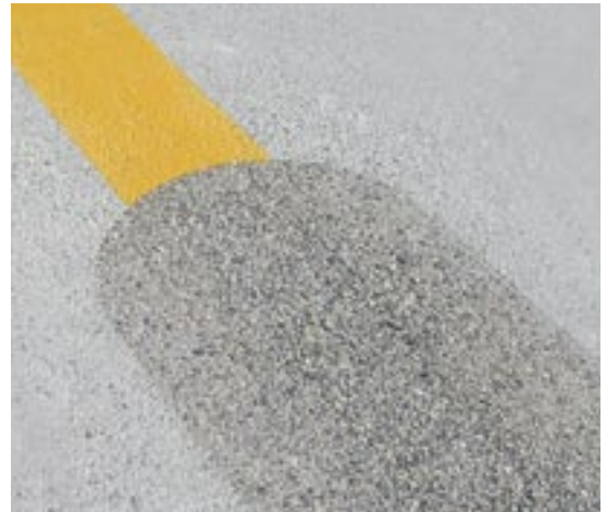
In one pass, markings are completely removed and the surface is prepared for recoating.
