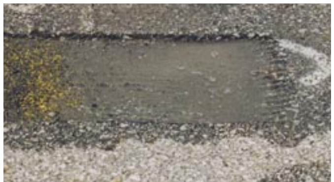
Grinding can leave ruts in the pavement as well as traces of striping.
